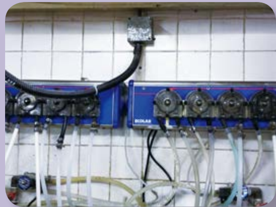
Cleaning chemical dispenser
