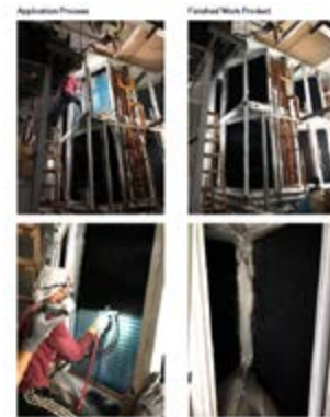
Conducted performance enhancement work of an air-cooled condenser at Regal Hongkong Hotel
