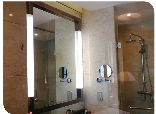
Regal Airport Hotel, Xi'an replaced the mirror lights of 297 guestrooms with LED lights to enhance energy efficiency.
