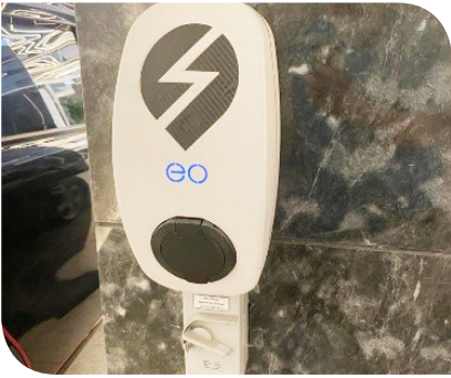
Electric vehicle charging station
